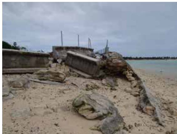
Photo 18: Structural failure (Credit: Shand)
