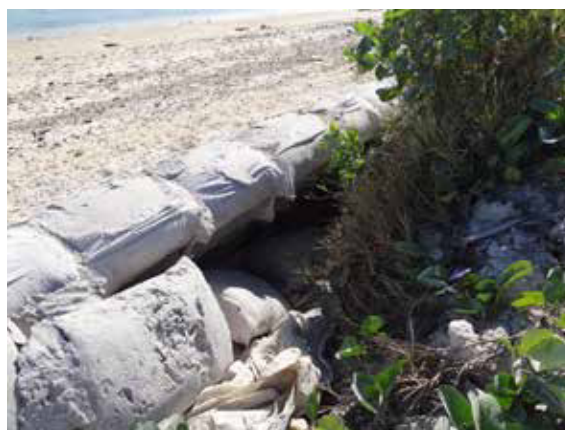
Photo 16: Overtopping (Credit: Shand)
