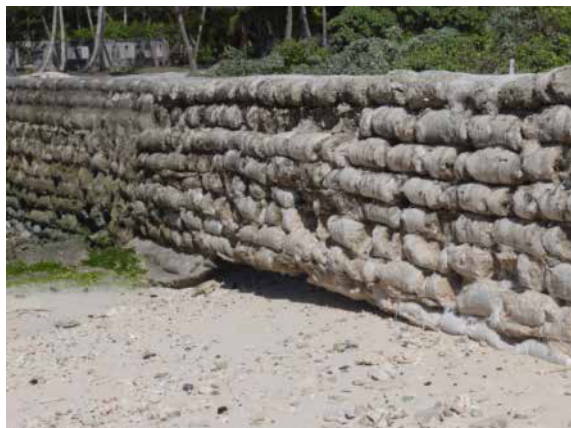
Photo 17: Undermining (Credit: Shand)
